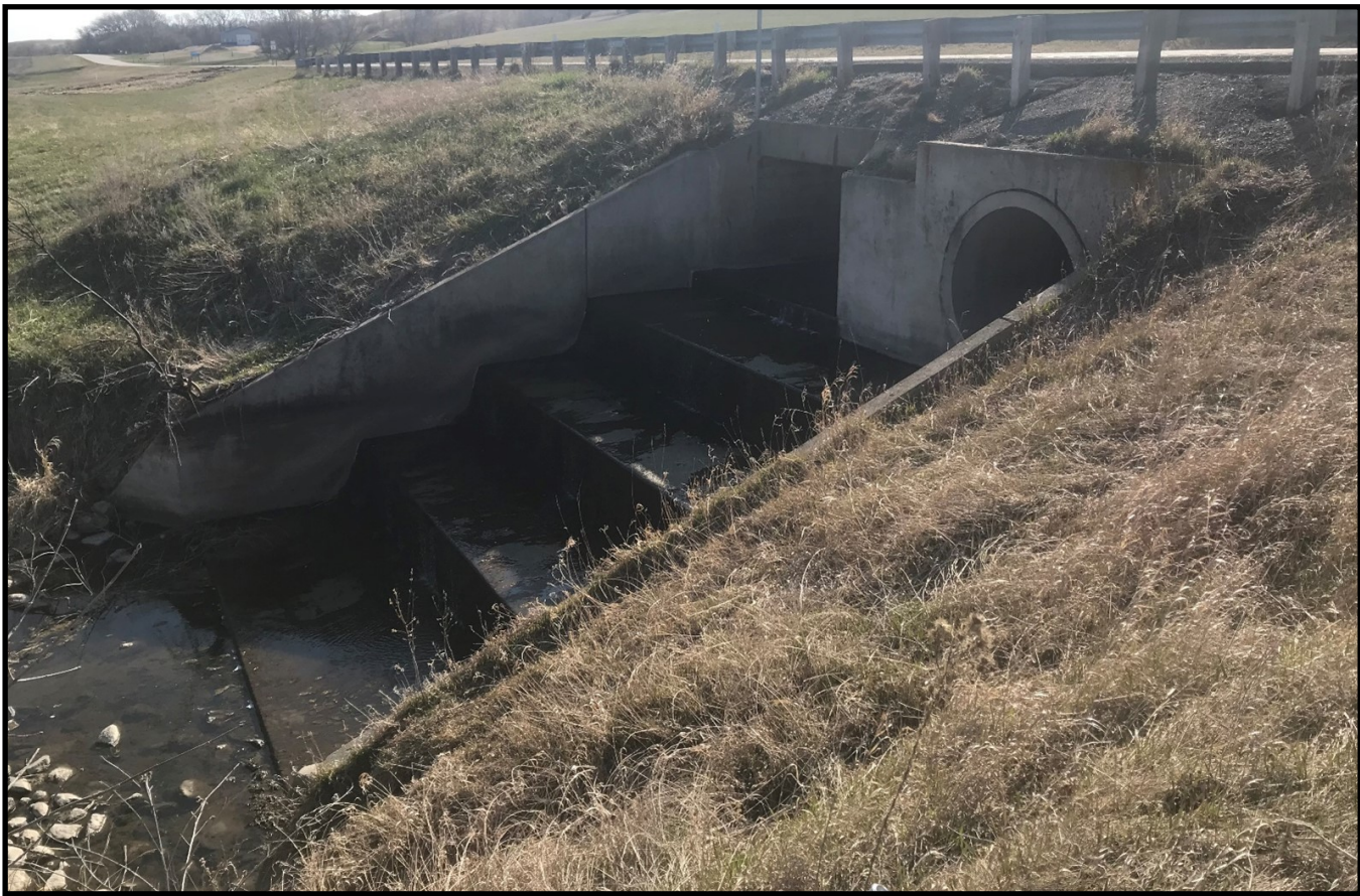
Minnesota State Highway 27 culvert. Photograph courtesy of Robert Sip, RRWMB Executive Director – April 22, 2021.
