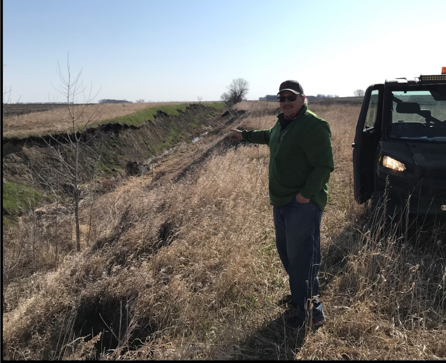
BdSWD Technician Troy Fridgen pointing out severe bank sloughing and erosion in the upper reaches of the Project watershed area. Photograph courtesy of Robert Sip, RRWMB Executive Director – April 22, 2021.
